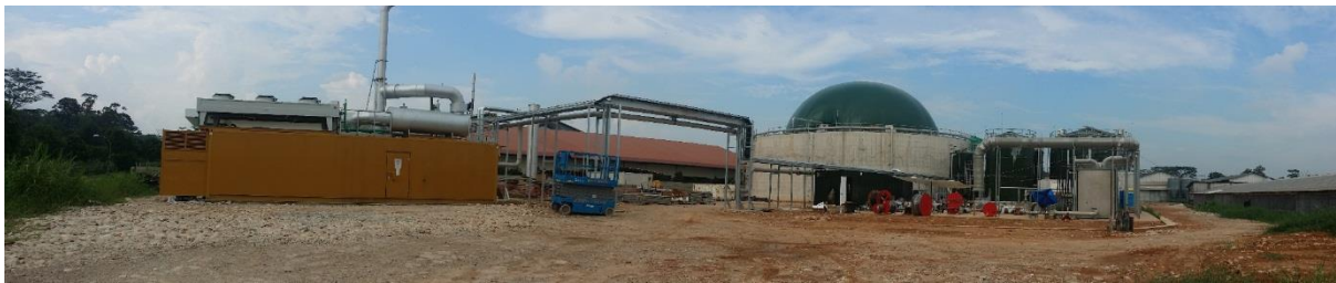
Figure 21: Anaergia SCCF Singapore project: Site overview.
