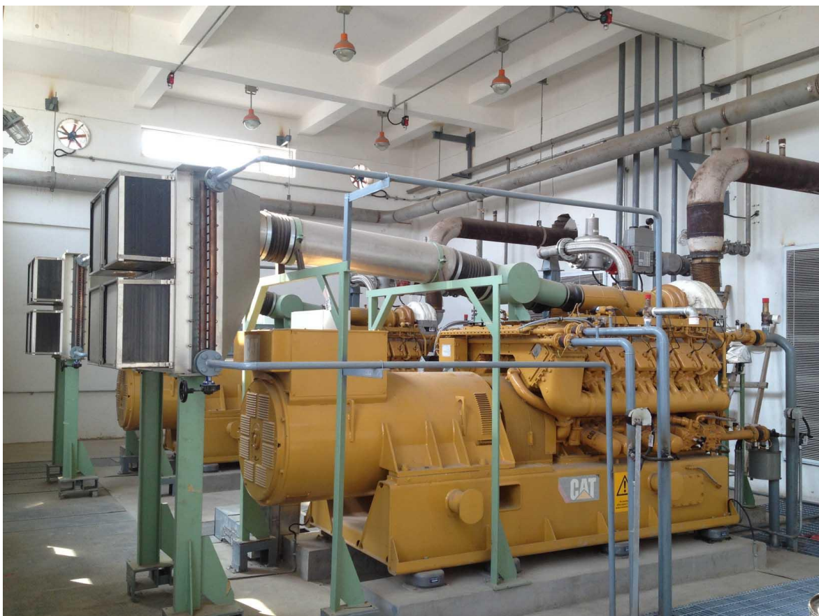
Figure 10: YFJA HeBei Province project: Cat CG170-12, 2x 1,200 kW biogas gensets view.
