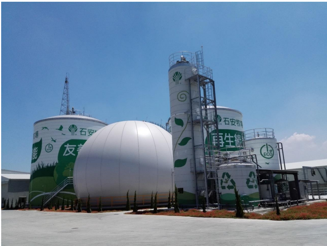
Figure 14: ShiAn Tainan Project: CSTR biogas system with double-membrane biogas storage and H 2 S scrubber system.
