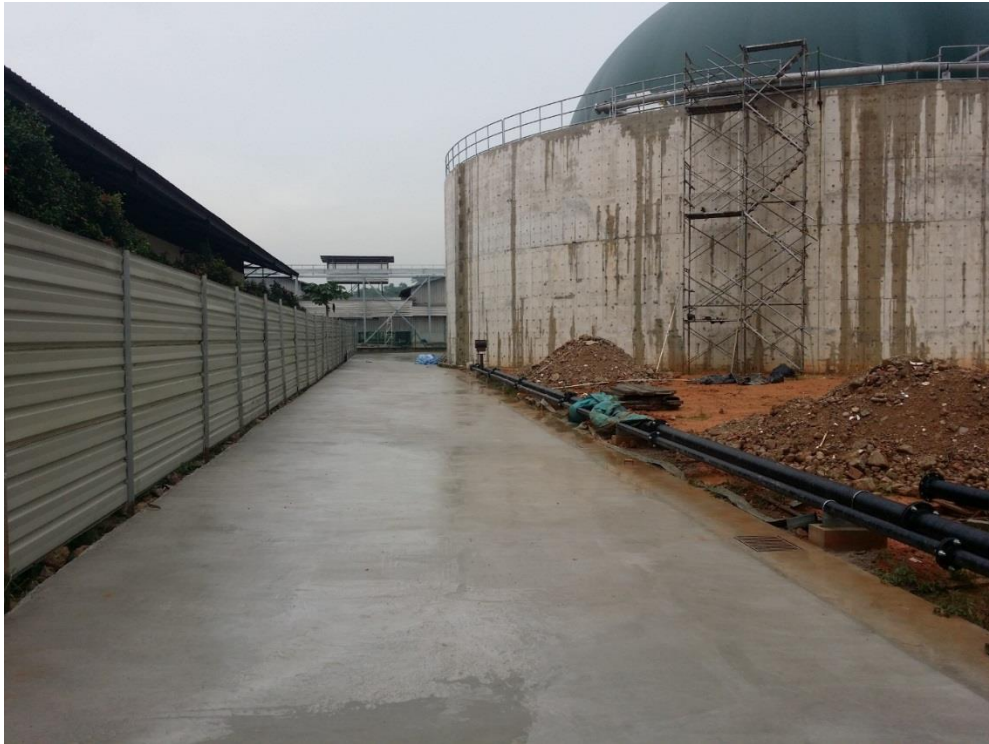
Figure 22: Anaergia SCCF Singapore project: Triton anaerobic digester is on the right.
