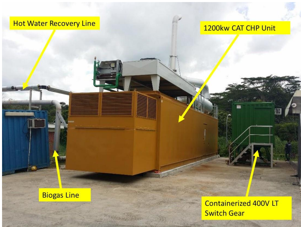
Figure 23: Anaergia SCCF Singapore project: Cat CG170-12, 1,200 kW biogas generator set in 85 dBA (1 m) sound enclosure with full CHP unit on top of the container.
