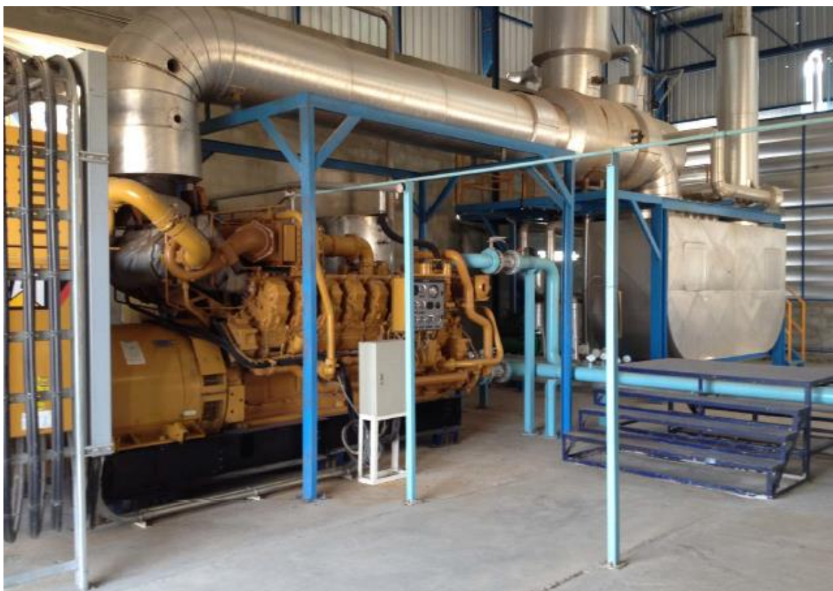
Figure 28: TQS Kanchanaburi project: Cat G3516A+, 1,100 ekW biogas generator set.
