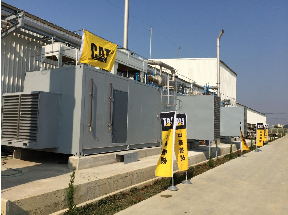
Figure 17: ShiAn Tainan Project: Cat CG132-08, 2x 400 ekW biogas generator sets in 54 dBA (10 m) sound enclosure.
