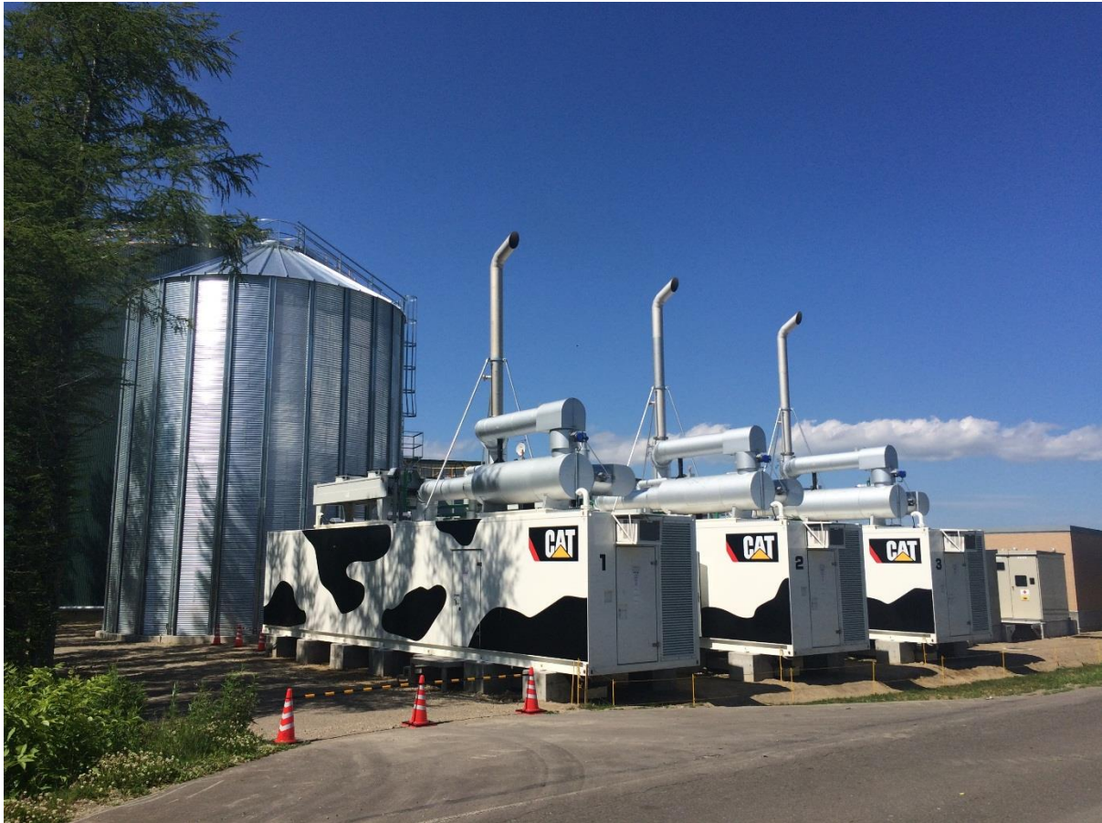
Figure 6: MES Hokkaido biogas-to-power project: Cat CG132-12, 3x 600 ekW biogas generator sets in containerized sound enclosure (85 dBA at 1 m).
