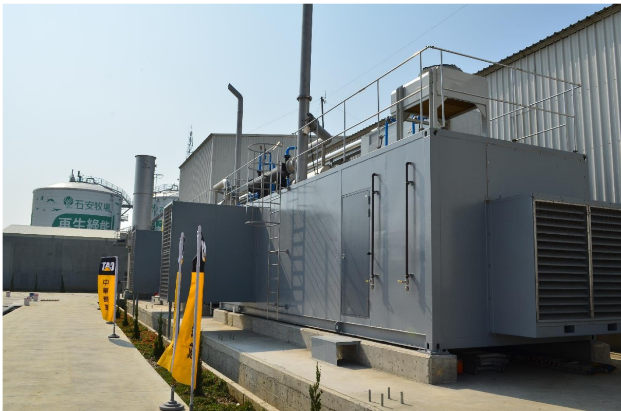
Figure 16: ShiAn Tainan Project: Cat CG132-08, 2x 400 kW biogas generator sets in 54 dBA (10 m) sound enclosure.
